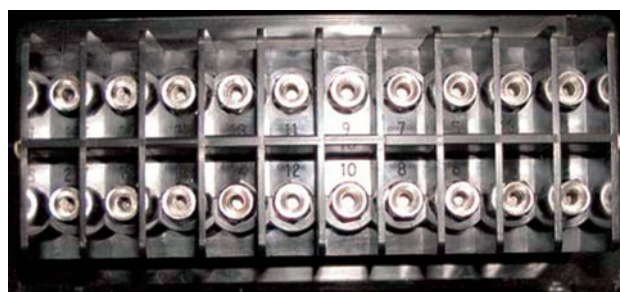
FT switch terminals 1 thru 20 (rear view)
